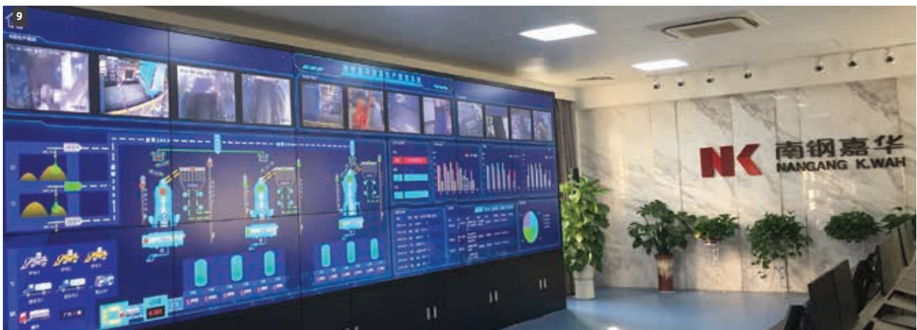
7: Jiangsu Huailong Smart Manufacturing Project Phase II (Control Centre Dashboard)
